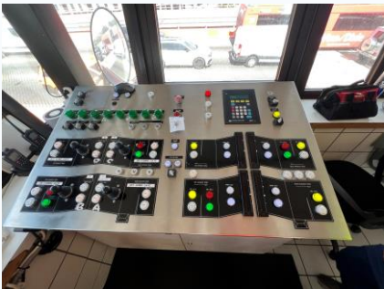
Obsolete Bridge Electrical Control System
