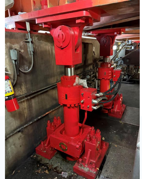
Hydraulic Piston Leaks
